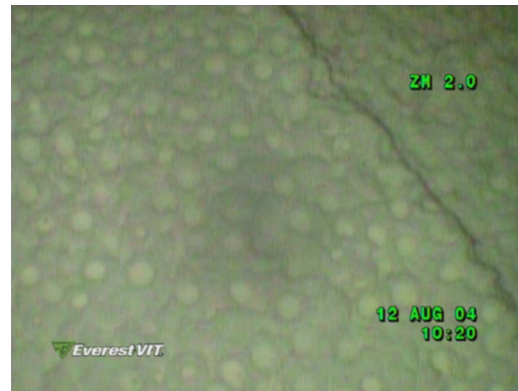
Fig. 19 Borescope image of oxide/oxide CMC outer liner with FGI after 10,667 h and 61 starts of engine test CT-7
