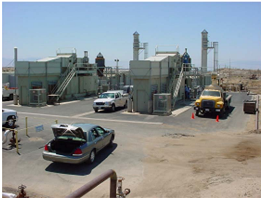
Fig. 3 The ChevronTexaco Bakersfield site with field test engine in package on the right
