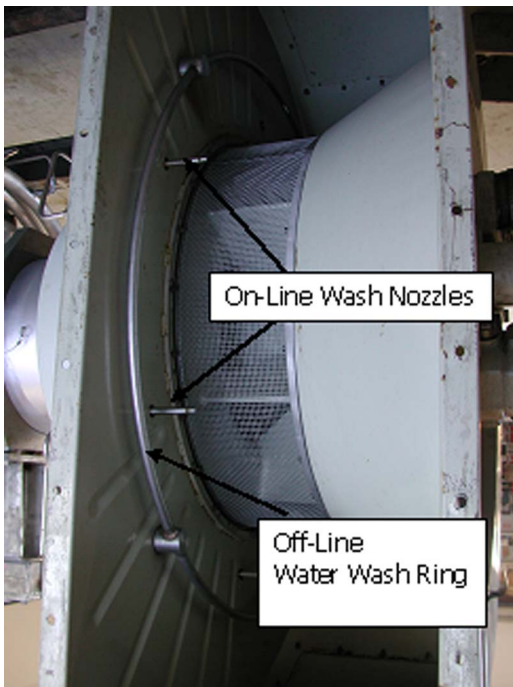
Fig. 7 Inside view of air plenum showing the off-line water wash ring and the on-line water wash nozzles
