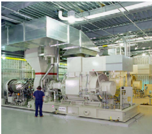
Fig. 4 Centaur ® 50S gas turbine engine at Malden Mills textile facility
