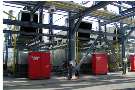
Fig. 8 Three Centaur-solar gas turbines
